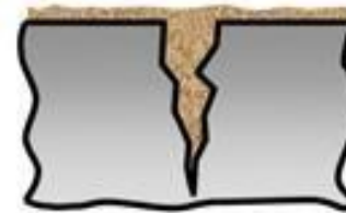
1 Crack filled with dirt
